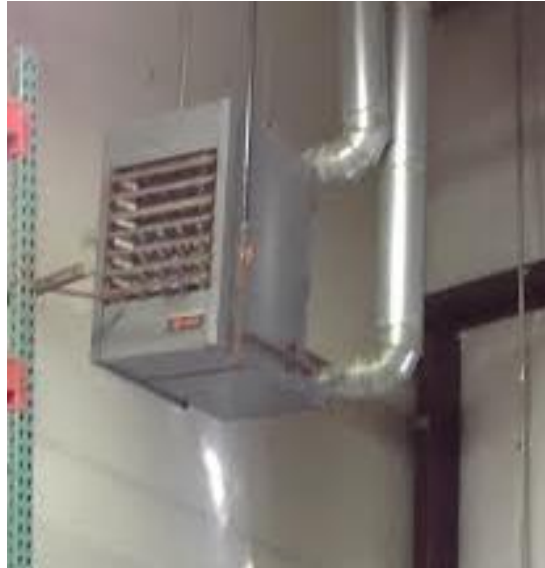
Figure 25: Physical Plant Warehouse Heating Unit
